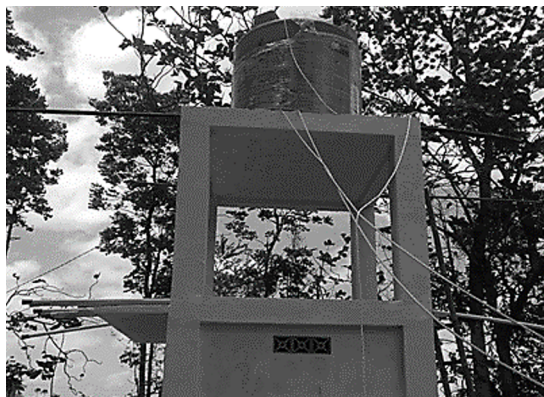
Fig. 7. The main water reservoir has a capacity of 5000 liters.
