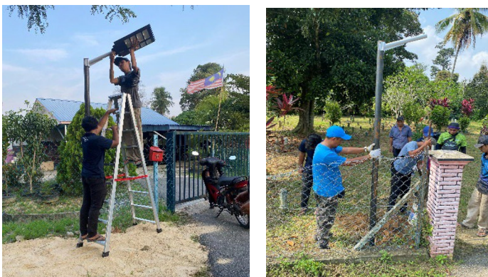
Fig. 2. Humanitarian activity by installing solar street light complete with pole
