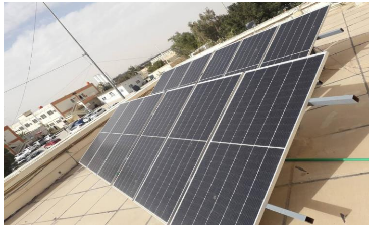
Fig. 5. Array of solar panel on building roof
