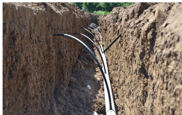
Fig. 1. Subsurface drip irrigation.
