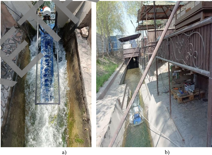
Fig. 3. View of the ditch a) and the installation site of the Archimedes screw turbine b)
