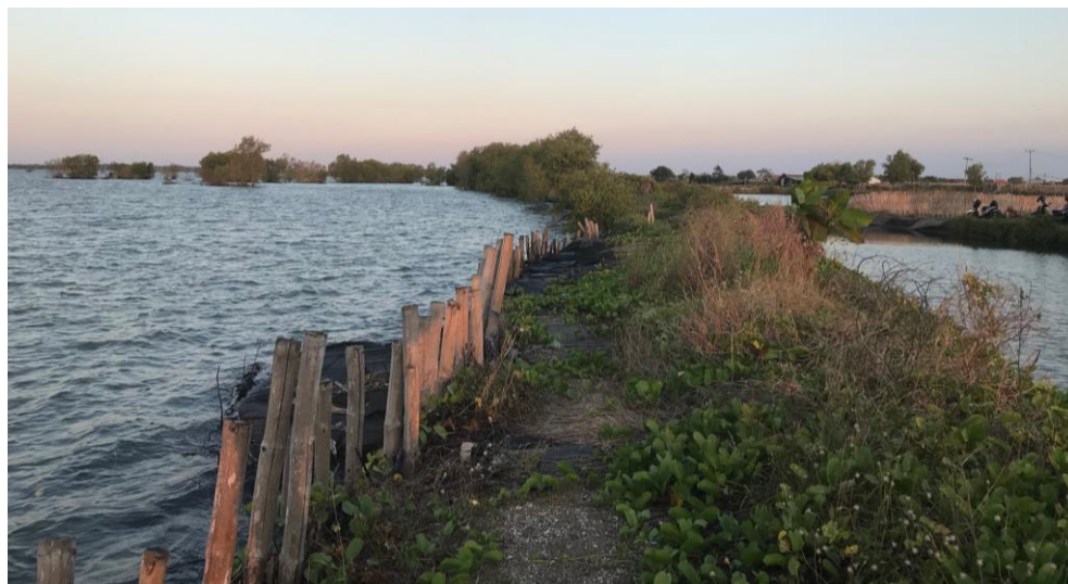
Fig. 11. Post-erosion coastal conditions
