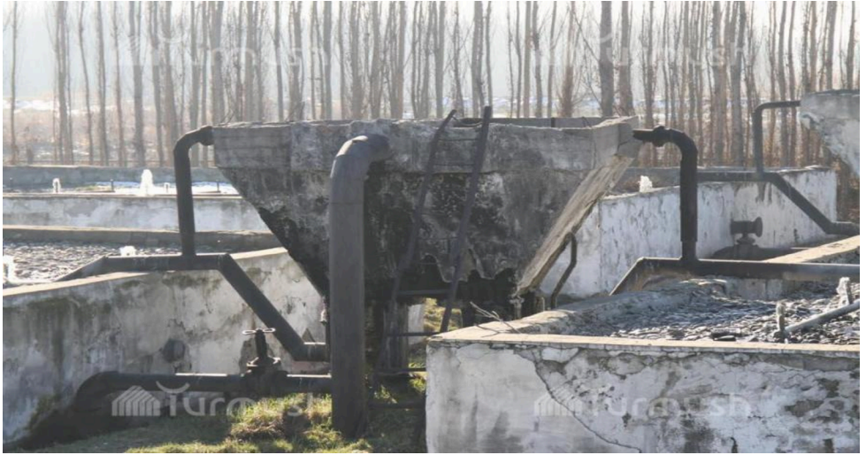
Fig. 5 Distribution bowl of biological filter treatment facilities in Jalal-Abad city
