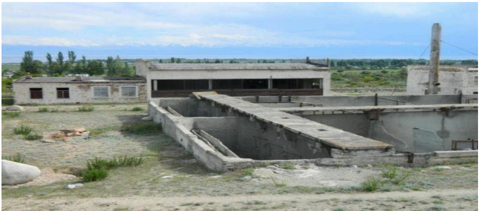
Fig.4 Biological water purification of the Cholpon-Ata wastewater treatment plant
