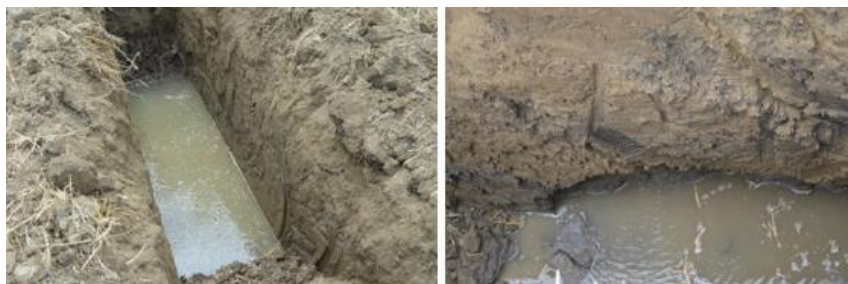
Fig. 2. The rise of the groundwater level in the arranged pits
