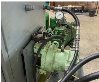
Fig. 3. Pump NAR 63/20 on a bench for testing throttle flow dividers/adders
