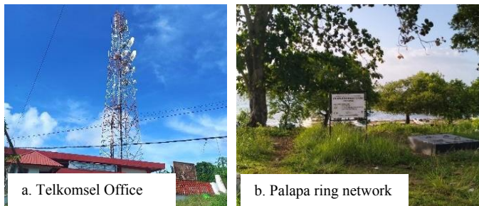
Fig. 11. Telecommunication facilities; a. Telkomsel office and b. Palapa ring network
