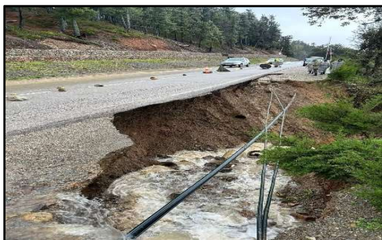
Fig. 13. Damage to road infrastructure between Tetouan and Chefchaouen on March 30, 2024
